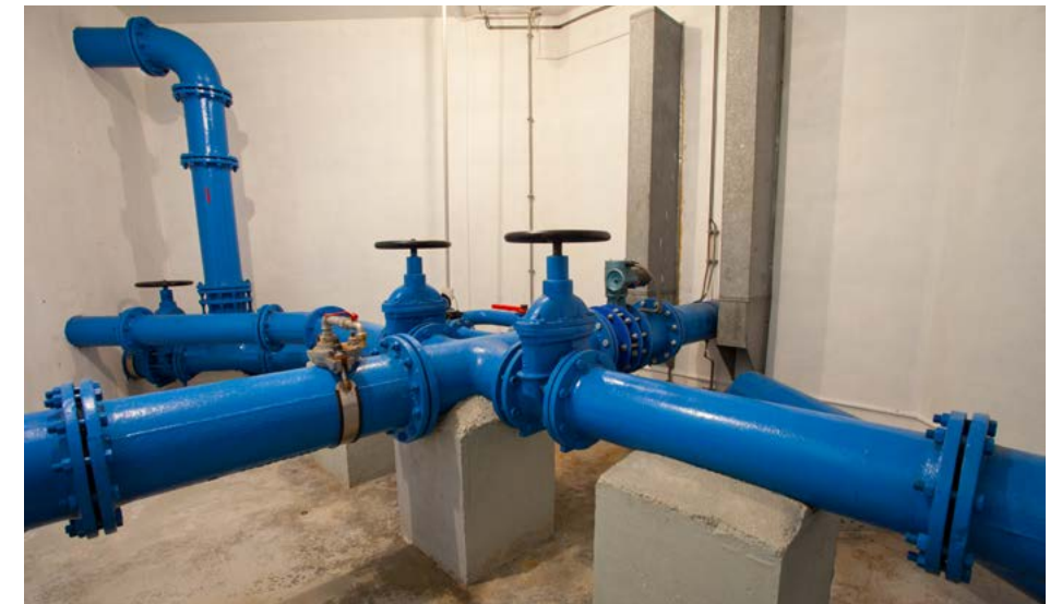
Armature v vodohranu
